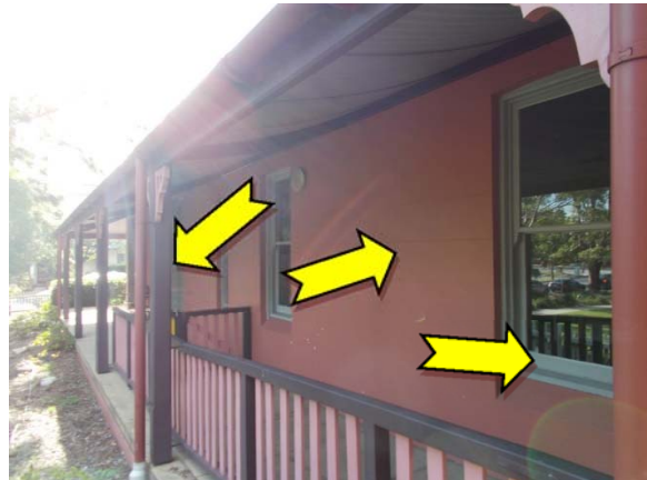
Photo 10. Exterior, throughout, walls and features – suspected pink, purple and green upper coloured paint systems.
