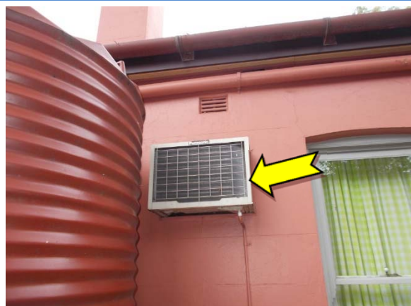
Photo 12. Exterior, south-west elevation, air conditioning unit, unknown refrigerant – suspected ozone depleting substance.
