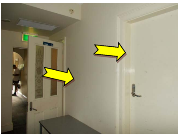
Photo 11. Interior, throughout, walls, doors and frames – suspected lead-containing cream upper paint systems.
