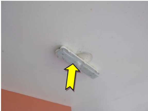
Photo 9. Interior, throughout, single tubed fluorescent light fitting – suspected PCB-containing capacitor.
