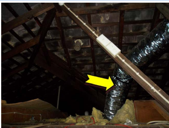
Photo 5. Interior, ceiling space, flexible ductwork – suspected SMF internal insulation material.
